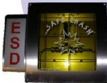
Pannello ESD ESD Panel
